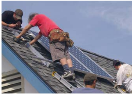
Installation of photovoltaic panels in Mission, BC Source: Vancouver Renewable Energy Co-operative
