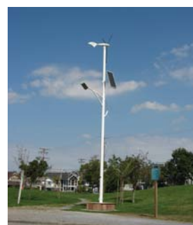
The City of Richmond is testing a new type of lighting system, generating both wind and solar energy, and storing the electricity to a battery to power the street light at night. Source: City of Richmond
