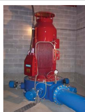
The District of West Vancouver is generating power from its drinking water system, with a 200 kW turbine that replaced a pressure-reducing valve.
